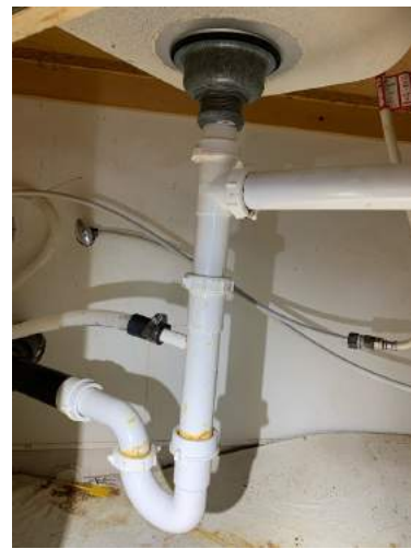
Plumbing: Under Cabinet
