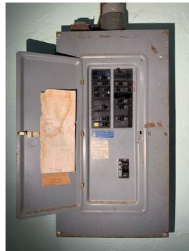
Electrical Main Panel
