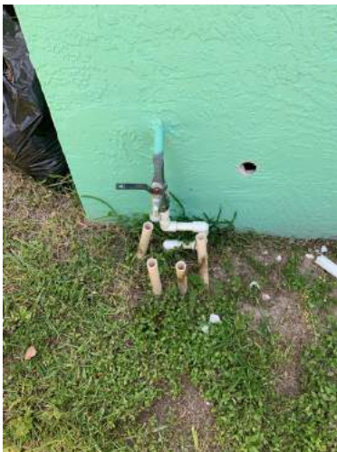
Water Supply, Main Shut-off, House Side
